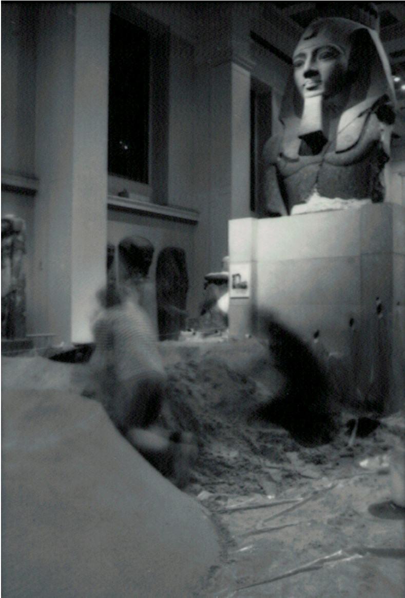
Figure 3.1 Photograph of the construction of Andy Goldsworthy's Sandwork at the British Museum, 22 October 1994. Photograph by and courtesy of James Putnam.
