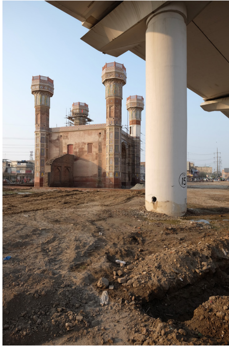
Figure 0.4 The Orange Line under construction around Chauburji gateway, 2019. Image by Chris Moffat.
