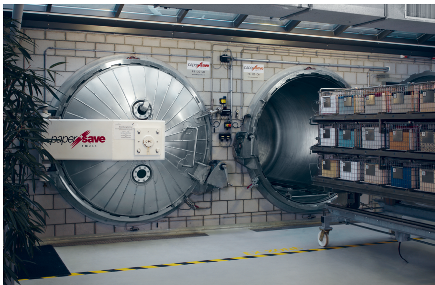
Fig. 1: The papersave swiss facility in Wimmis on the premises of the Nitrochemie Wimmis AG, in operation from 2000 to 2022. Interior of the papersave swiss facility. The treatment chambers. Photo: Nitrochemie Wimmis AG
