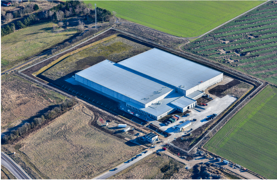
Fig. 3: The building site for a new storage facility in Vinge. Photo: DS Flexhal
