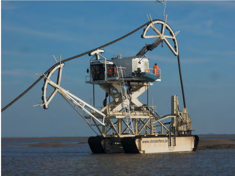
Fig. 1.1: This modern submarine cable trencher, a special machine for laying undersea cables offshore, weighs more than 100 tonnes.
